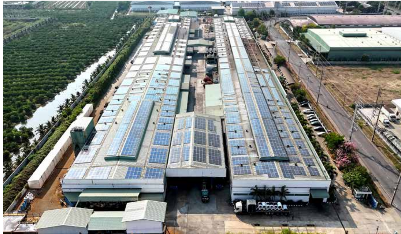
Solar rooftop plant at Rajratan Thai Wire Co. Limited, Ratchaburi, Thailand
